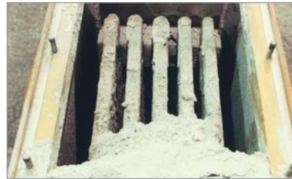
Fig. 2a: Bag air filter (intake side)
