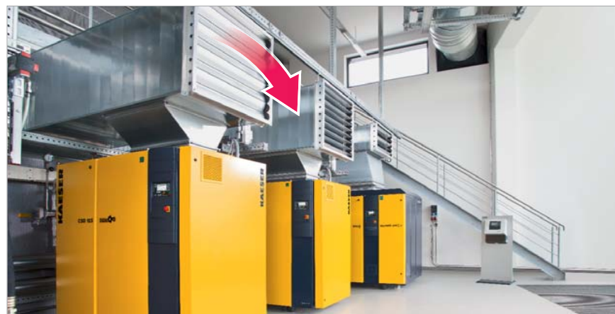
Fig. 3: Compressed air station with thermostatically-controlled air ducting
